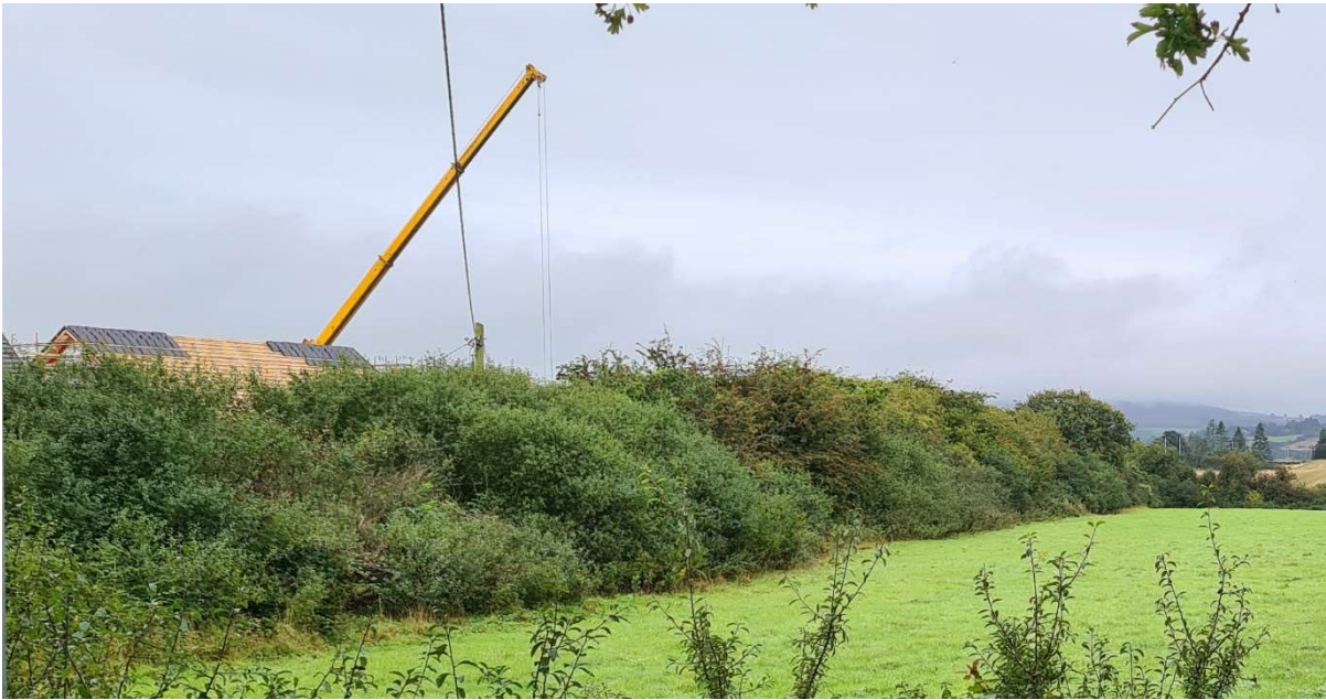
Looking east on to the existing hedgerow between the development site and Hazelbrooke with more advanced construction
