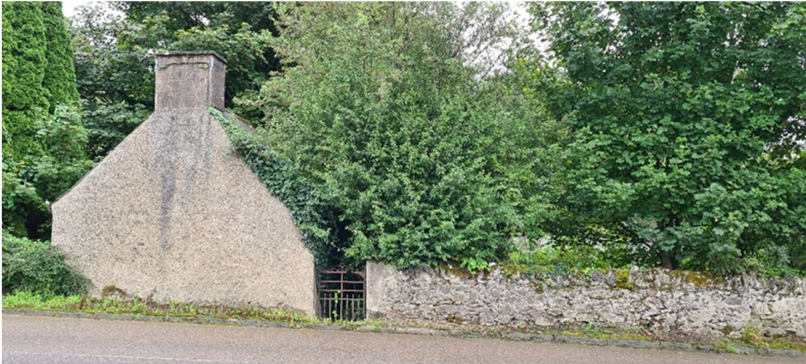
The gable end of the derelict cottage together with a pedestrian gate and limestone rubble walling standing on the carriageway edge of the Ballyvinitter Road.
